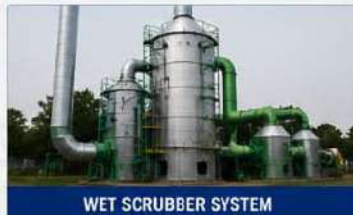
WET SCRUBBER SYSTEM
